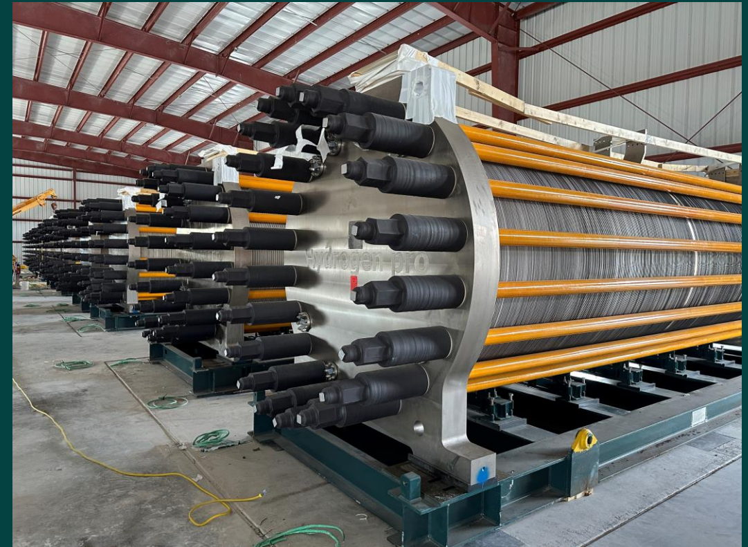
HydrogenPro electrolysers at the ACES project site in Utah, US
